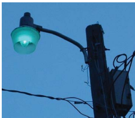
Mercury Vapor Lamp
