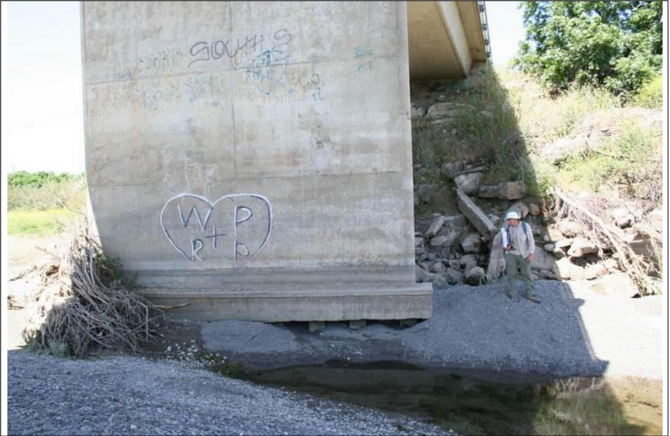
Figure 14 Bridge pier erosion at Esparto Bridge
