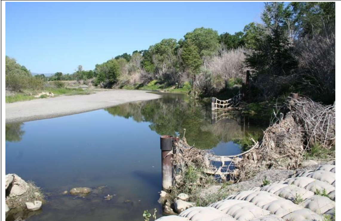
Figure 2 Palisades with debris north bank
