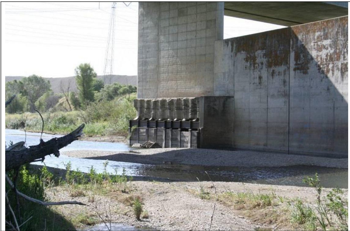
Figure 16 Highway I-505 Bridge - Evidence of two-stage building Former degradation as accounted-for in second stage
