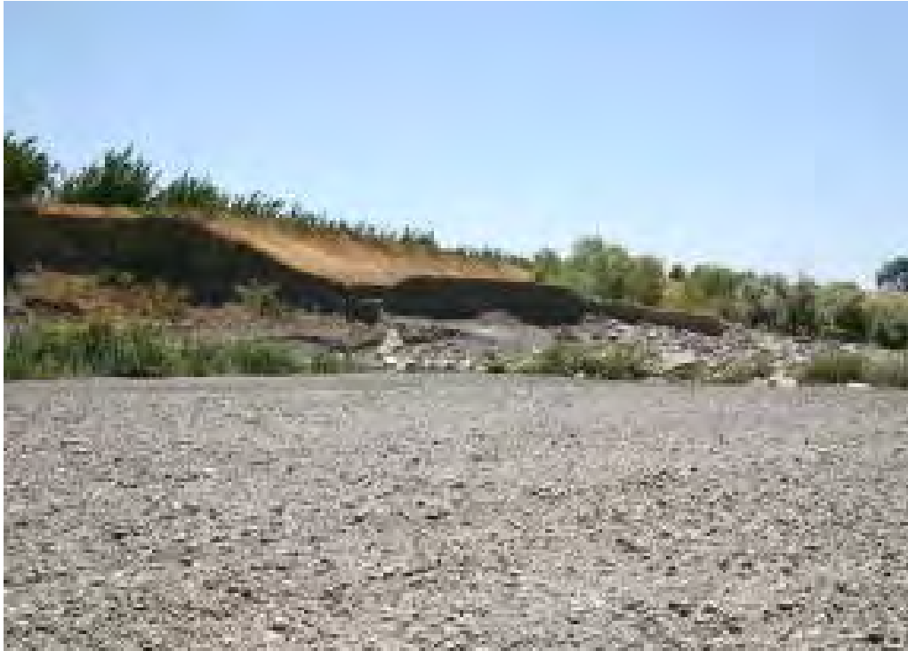
Figure 35 Active erosion of upstream spur dike, RM 21.55 north bank (2008).
