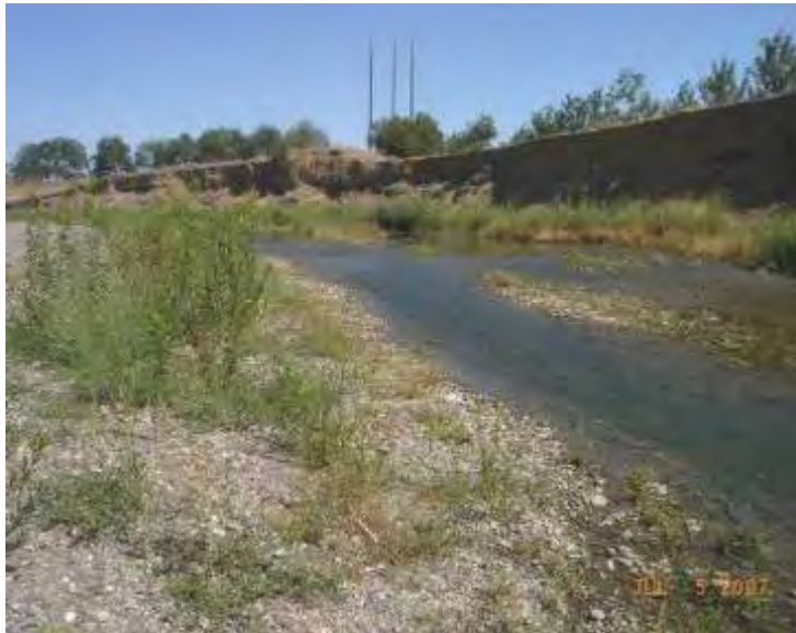
Figure 33 Bank erosion at the outside bend of the meander near RM 21 (2008)
